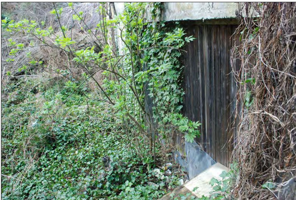
Figure 15 Below: View of basement level enclosure and ravine at east side of building (April 2011)
