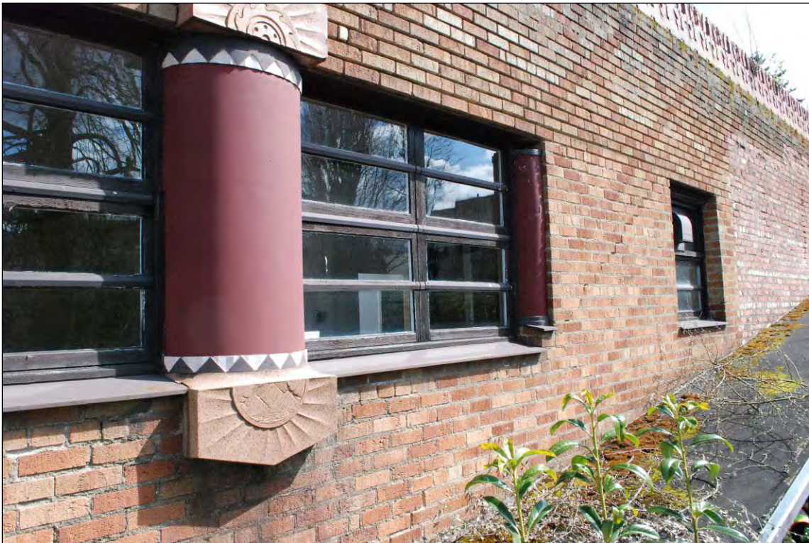
Figure 13 Below: Detail view of second level wood windows, with painted metal columns and decorative terra cotta pieces (April 2011)
