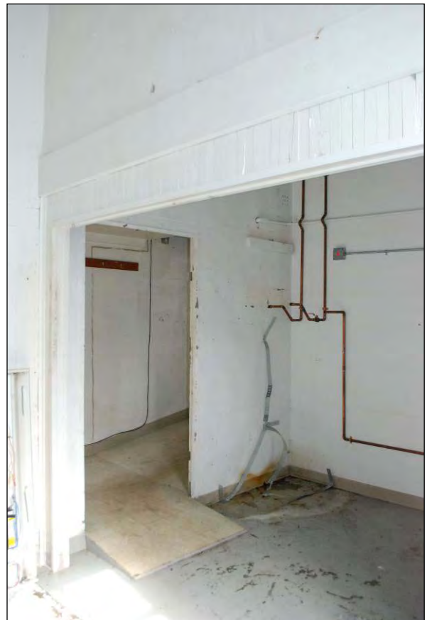
Figure 31 Below: View of ground floor ramp from down to southeast corner of building, looking west (April 2011)
