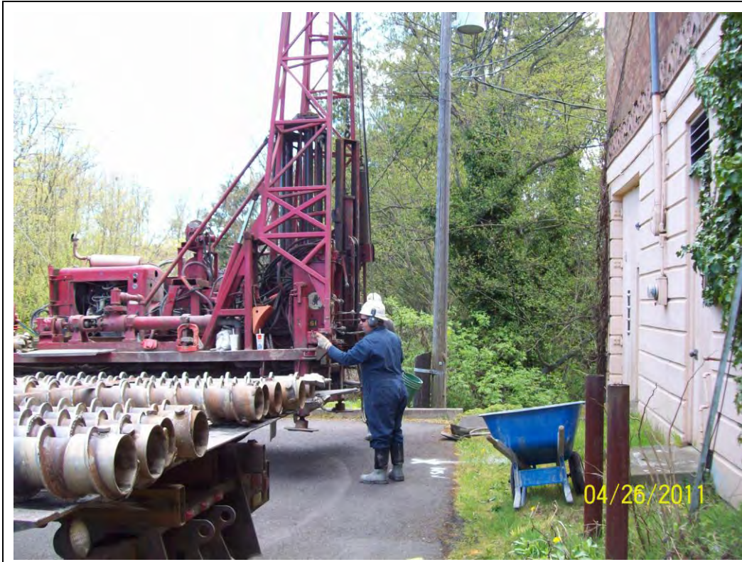
7. Borehole B2, also advanced to 50 feet bgs, was on the east side of the building, adjacent to visible building settlement.
