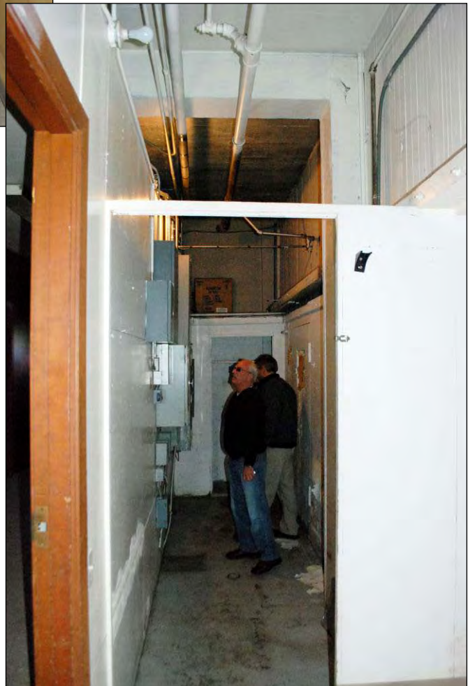
Figure 23 Below: View of utility corridor on ground floor, between main east and west areas of building, looking north (April 2011)
