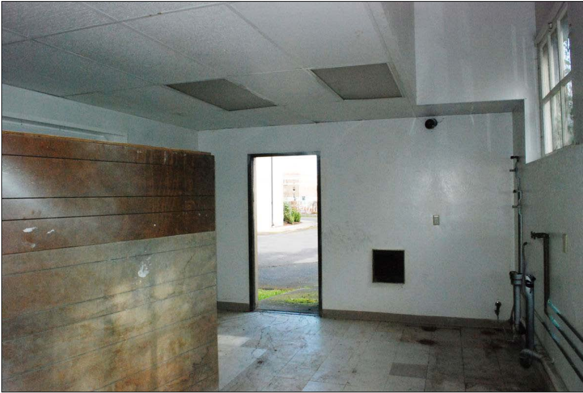
Figure 28 Above: Overall view of storage room at northeast corner of ground floor, looking north (April 2011)
