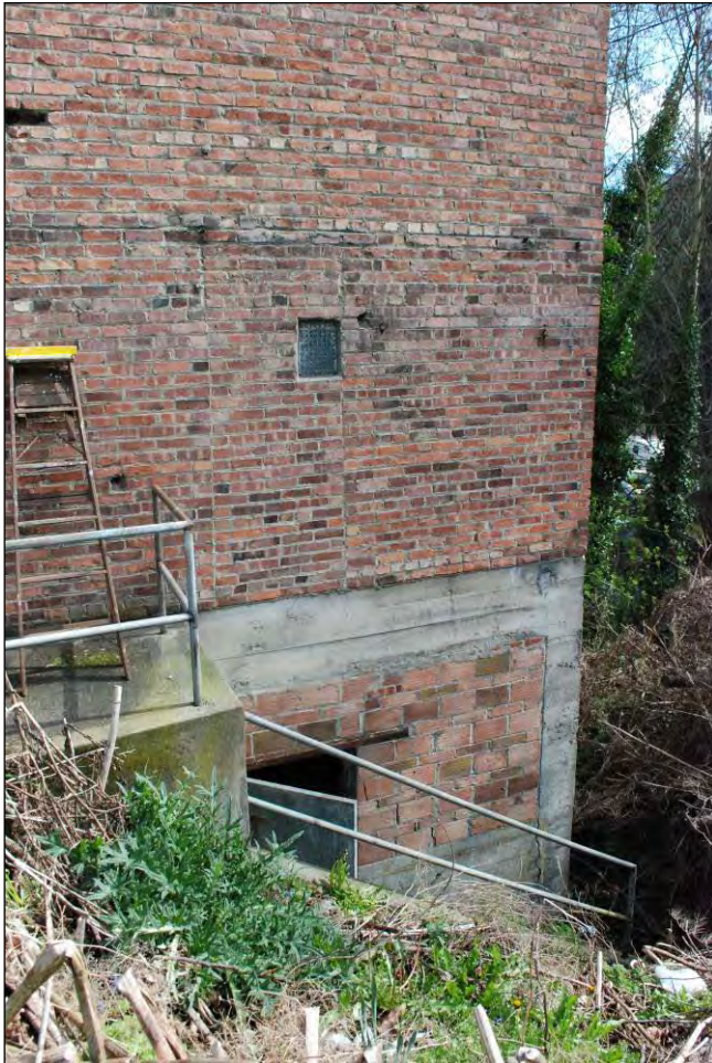
Figure 14 Left: View of entry to basement, at southeast corner of building (April 2011)
