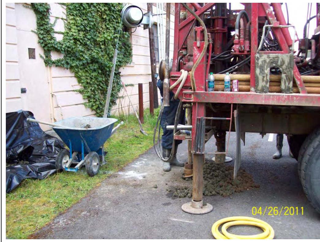
8. Soil profiles were very similar in both of the boreholes, with very soft and soft clays encountered to depths of approximately 30 to 35 feet. Note bedding clay cuttings.
