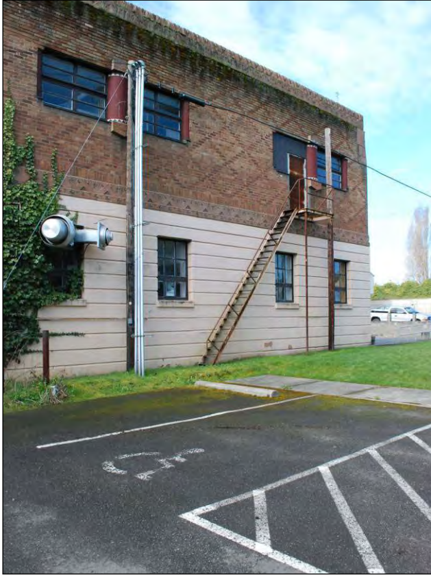
Figure 10 Left: Detail view of fire escape, looking across the parking lot north of the building towards the west (April 2011)
