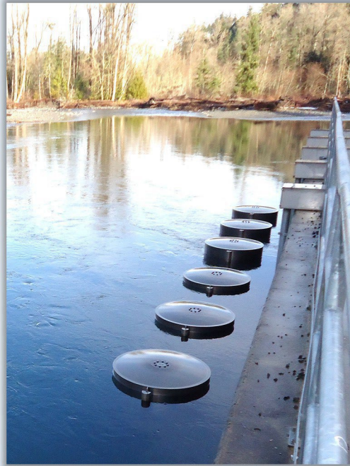
Elwha Surface Water Intake Screens
