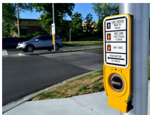
Figure 2-16 “H-style” (above) and APS-style pedestrian pushbutton (below)
