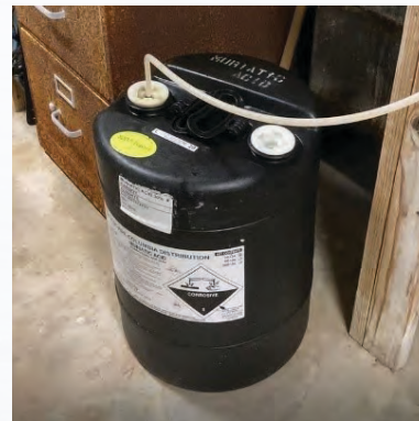
After: The new vapor-tight connector from the acid drum to the feed line.
